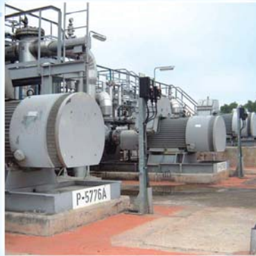
Application on LWSR pumps (before)
