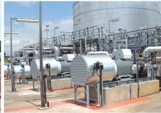
Application on LWSR pumps (after)
