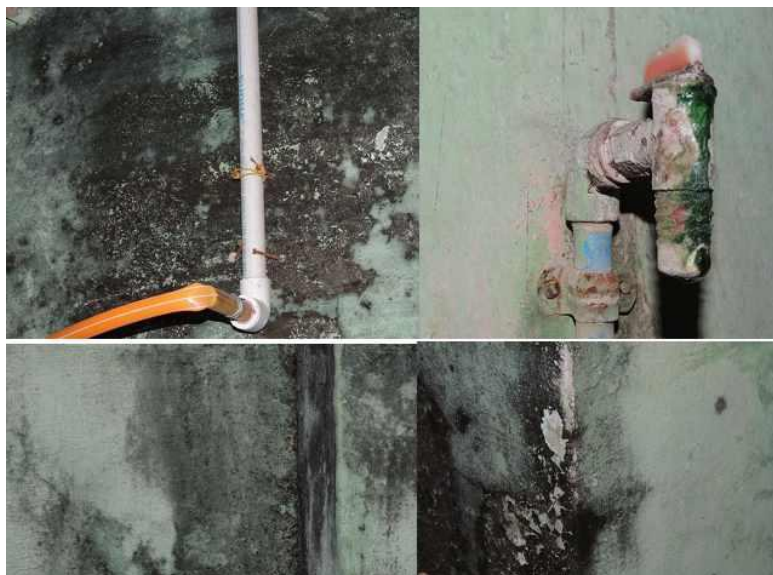
Plate 1 Photographs shows the algal patches on the wall of the buildings and other structures in different stations of the Visakhapatnam
