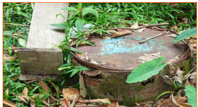
Figure 3. The steel drum barrel that served as a septic tank
