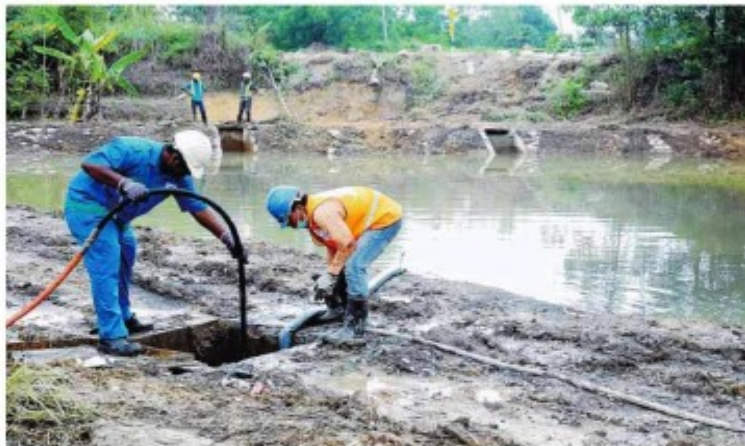
Indah Water Konsortium employees cleaning the sewerage system at the oxidation pond. — Picture by Syazana Rose Anwar
