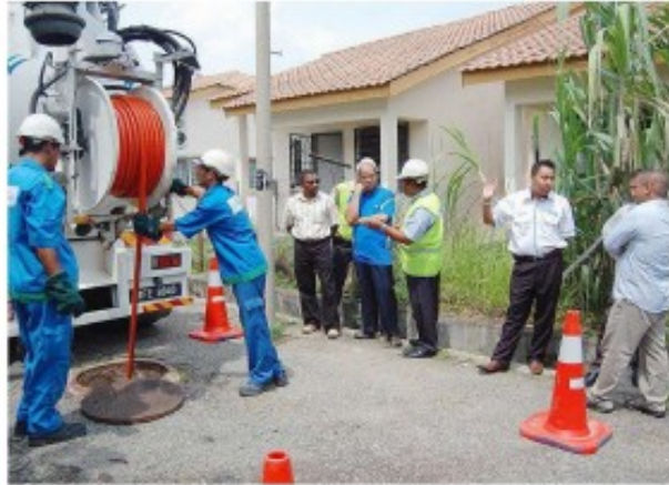
Getting the job done: IWK workers clearing out the sewage system as some residents look on.
