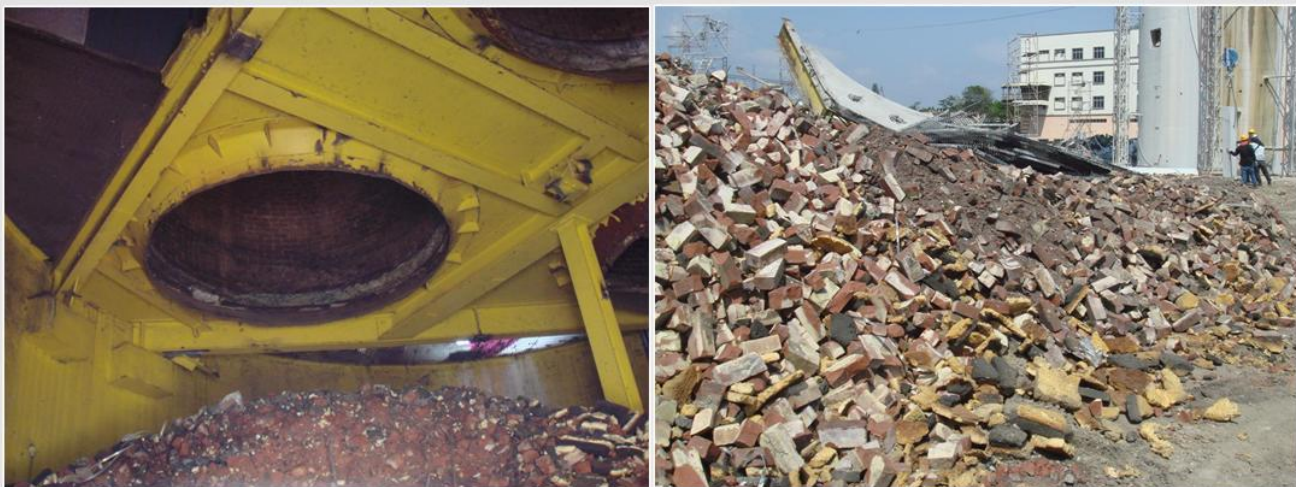
Figure 7: Brickliner from the Demolished Chimney Potentially-Contaminated with Heavy Metal Ash (SW 104) Due to Close Contact Throughout Plant's Operational Lifespan
