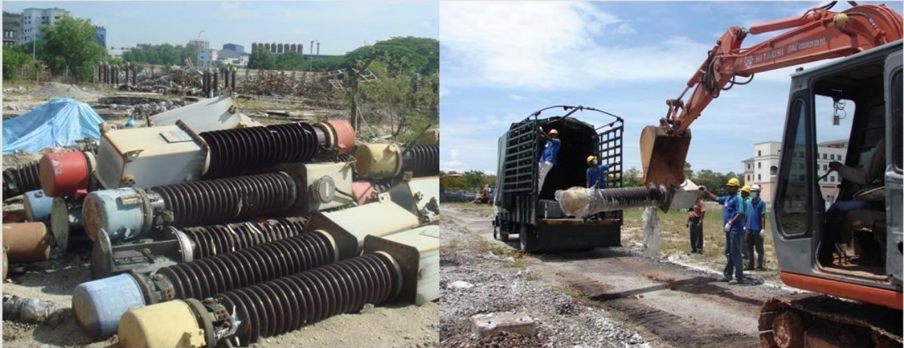
Figure 8: Transporting the Oil-Filled Circuit Breakers Declared as SW 409 to Prescribed Premises for Recycling and Recovery Process
