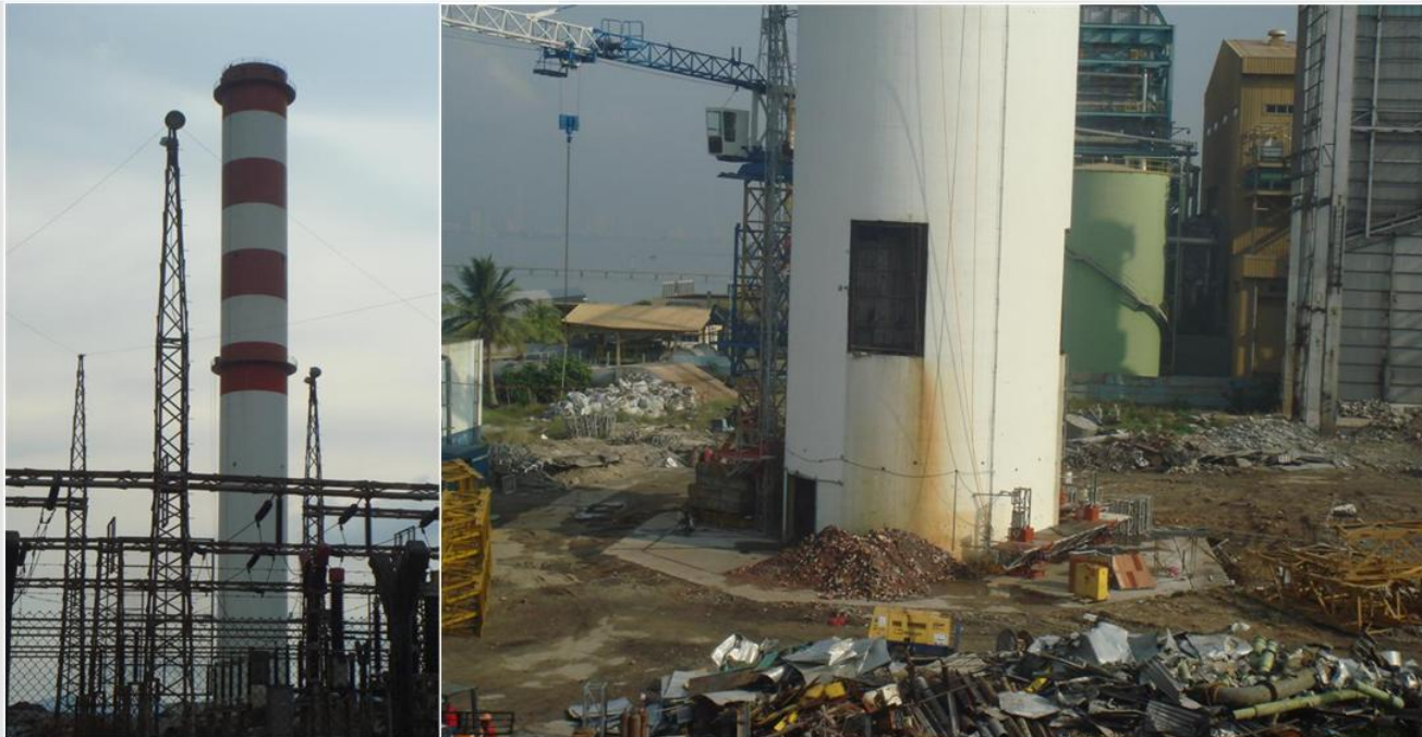
Figure 6: The 110 m Tall Chimney Contained in Windshield
