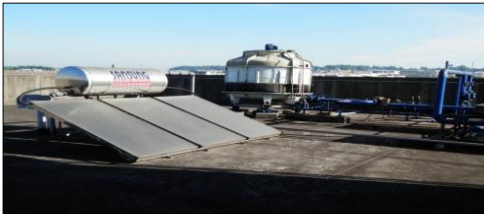
Figure 29: Solar panel at rooftop of staff hostel.
