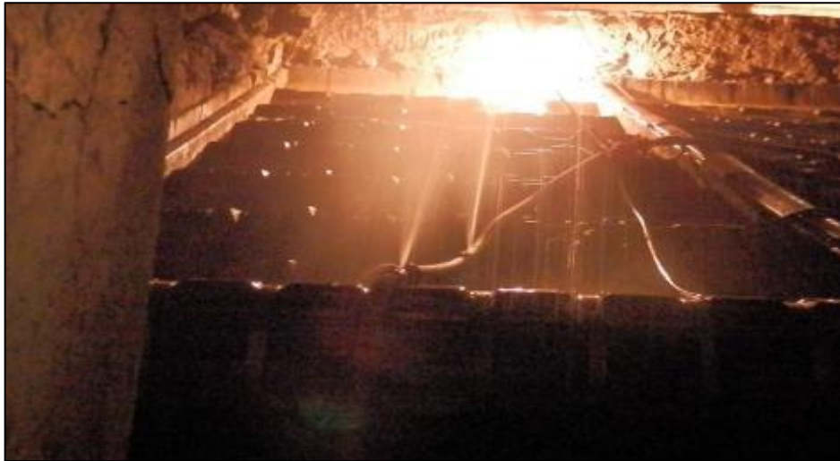
Figure 15: Grates inside furnace, maintenance is being done to clean up the furnace.
