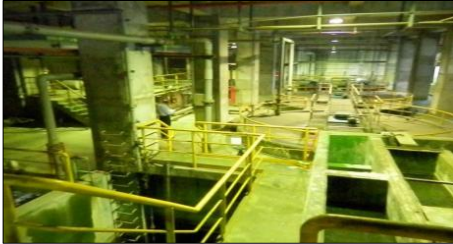
Figure 19: Waste Water/Leachate Treatment Plant
