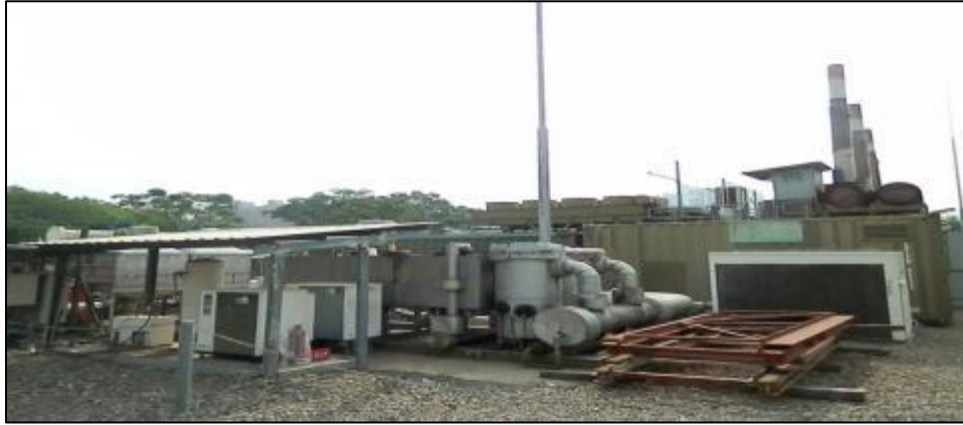
Figure 33: Methane Gas Power Plant
