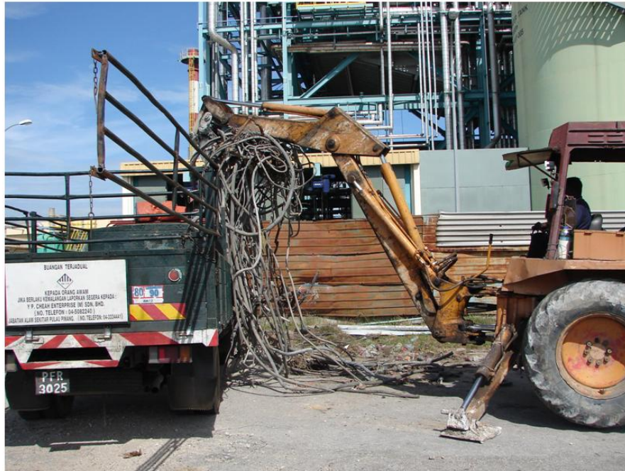
Figure 4: Electrical Cables Shall Be Disposed to Prescribed Premises Licensed for Scheduled Wastes Code SW 110 (Partial or Full Recovery)
