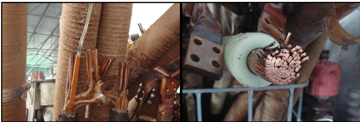
Figure 1: Precious Metals (Copper) Contained within the Electrical Cables and Assemblies
