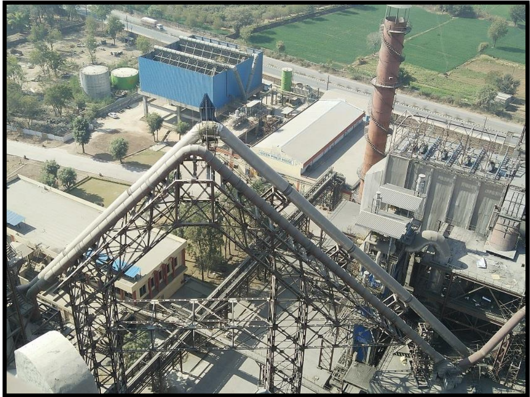
Hot air Recirculation duct connecting to Waste heat recovery system (WHRS)
