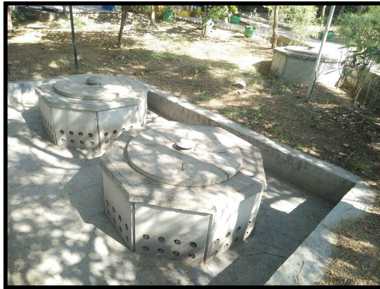
Rainwater harvesting unit
