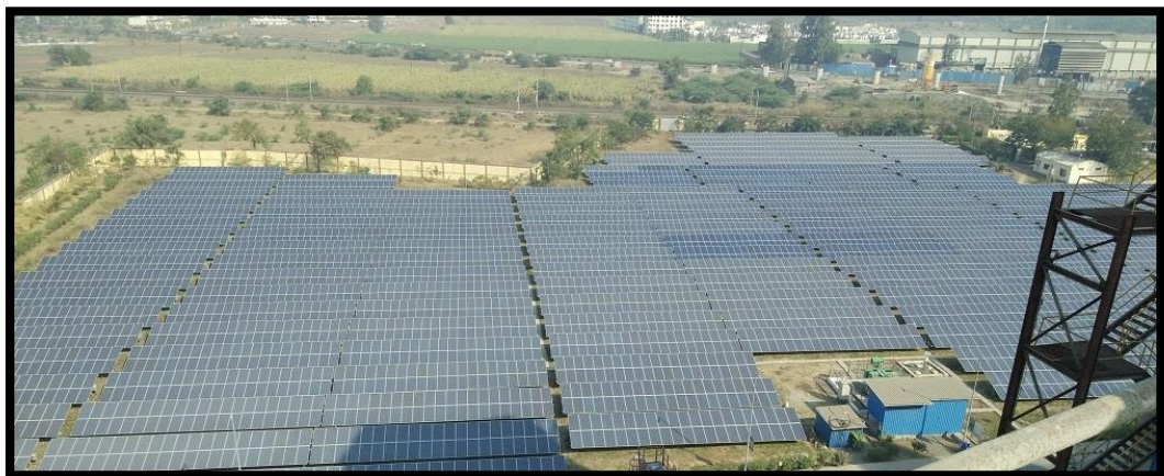
2.4 MW Solar Power generation plant at JK Lakshmi Surat Grinding Unit
